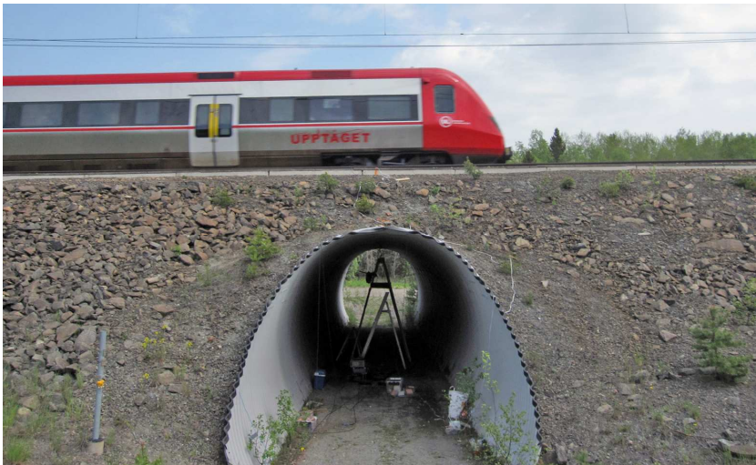
Figure 1. View of the bridge during the passage of an X52 commuter train
