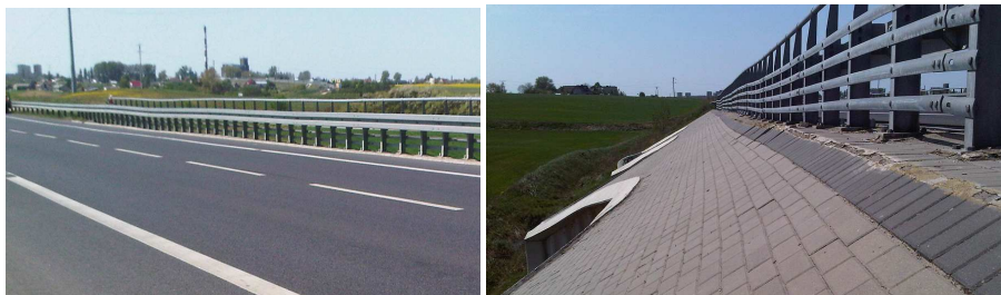
Figure 5 View of deformed parapets
