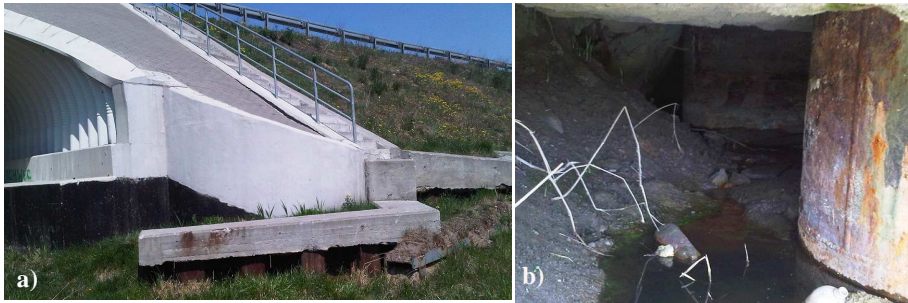
Figure 4 a) View of concrete beams placed on Larsen steel piles (walls) at the bottom of the embankment; b) view of space under pile capping
