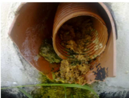
Fig. 6 Outlet of drain with fine particles that are washed - out from the backfill
