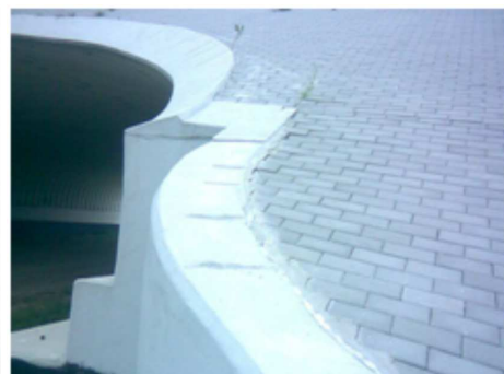
Fig. 7. Visible settlement of paved bevel end of the bridge
