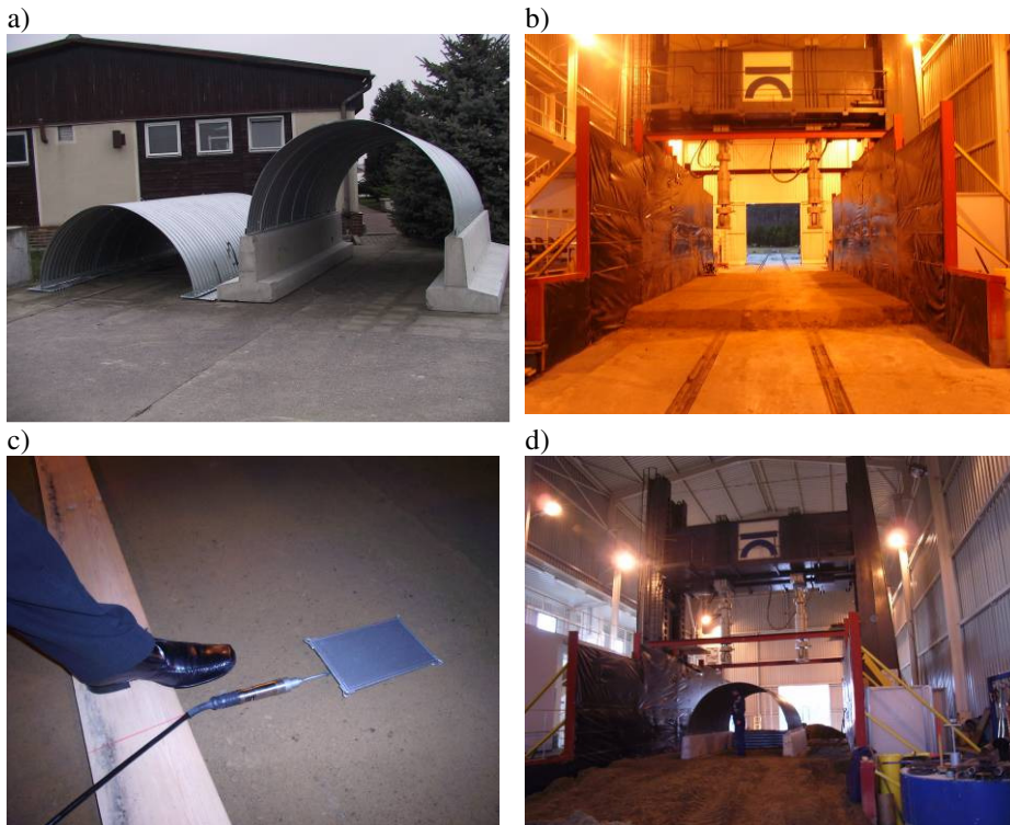
Figure 4. a) HelCor steel arches delivered to Roads and Bridges Research Institute; b) first compacted soil layer c) earth pressure cell used for measurement of soil stress under foundation. d) corrugated flexible structure settled on rigid concrete foundations at the stand
