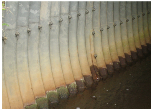
Figure 2. Typical rust in water line after 30 years
